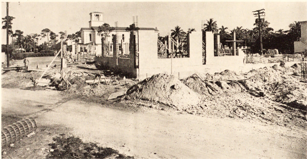
Barry's new student center and dormitory are taking shape as construction progresses to meet a fall, 1962, deadline.
