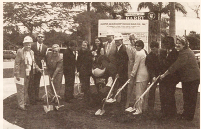
Barry Student Services leaders break ground for the new building (Photo by Dadi Rafnsson)
