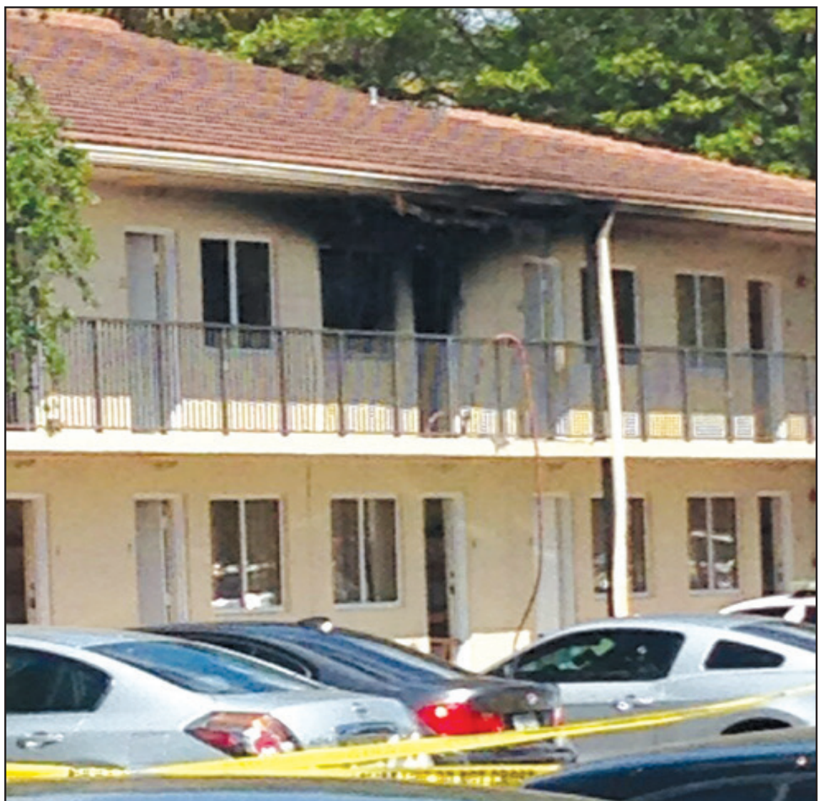
The aftermath of the fire in room 34 of Browne Hall.
